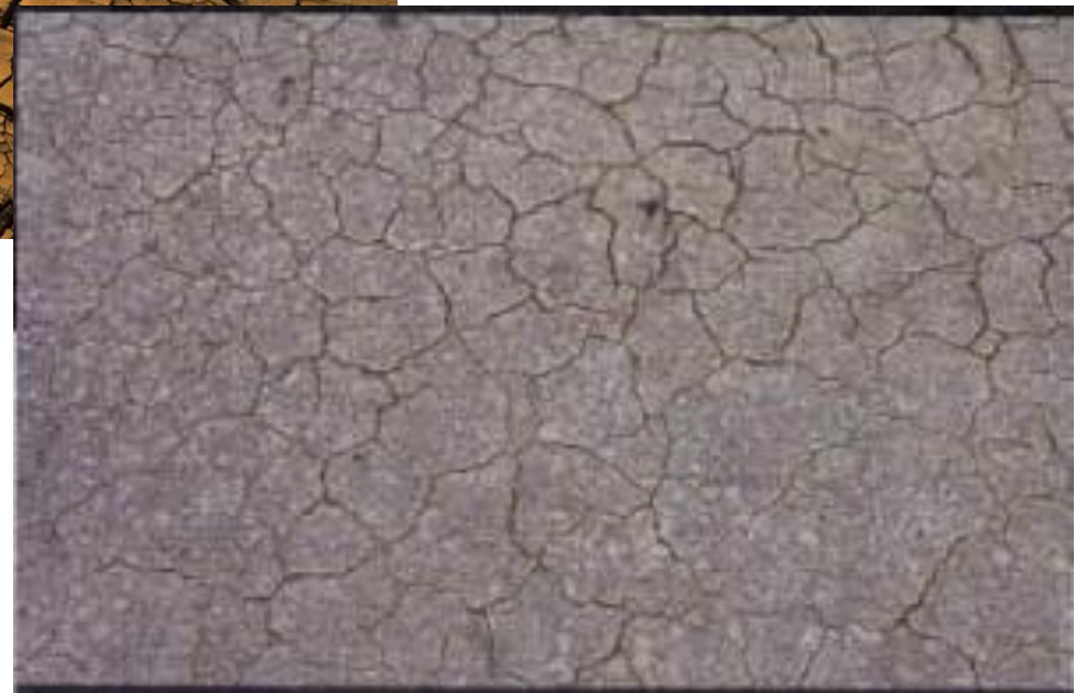
1. Plastic Shrinkage Cracking
